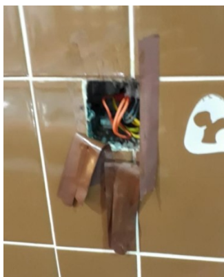
< Covers missing from socket sin Pool/Wet change side
