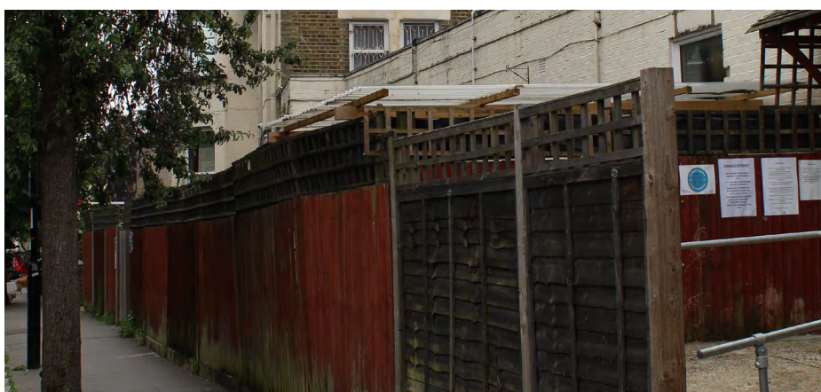
134. Loss of historic boundary treatments and use of modern materials for boundary walls
